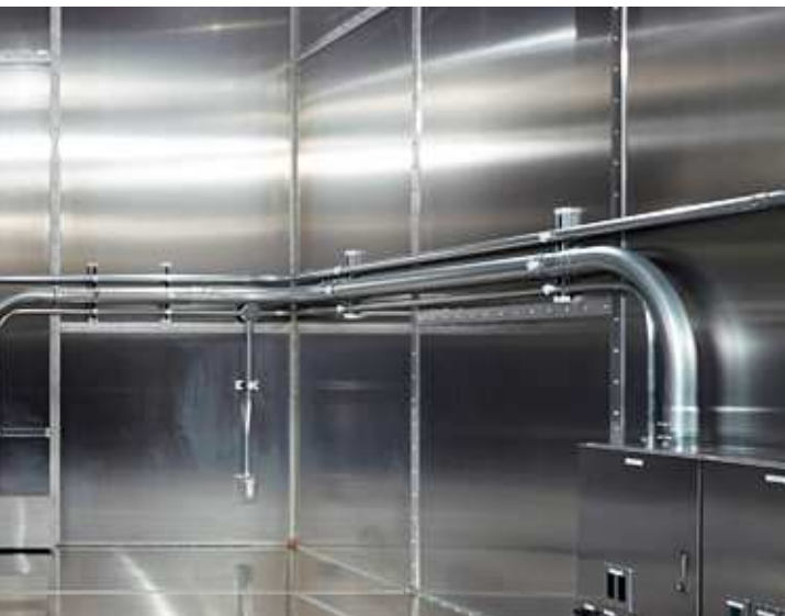
Large-area shielding of a transformer station using Aaronia Magnoshield® DUR panels.
